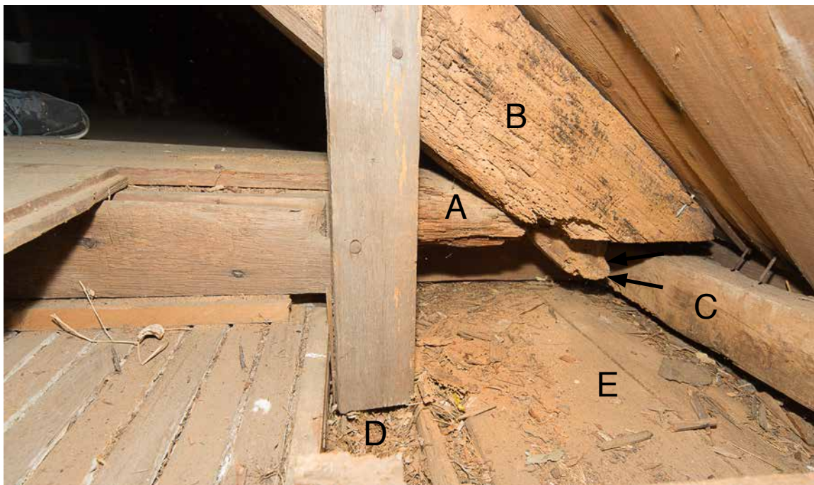
Photo 26: Photo of the end of the northerly chimney girt taken in 2016. The boards forming the cornice soffit are marked "E". As at the northerly chimney girt, current conditions are unchanged from 2005.
