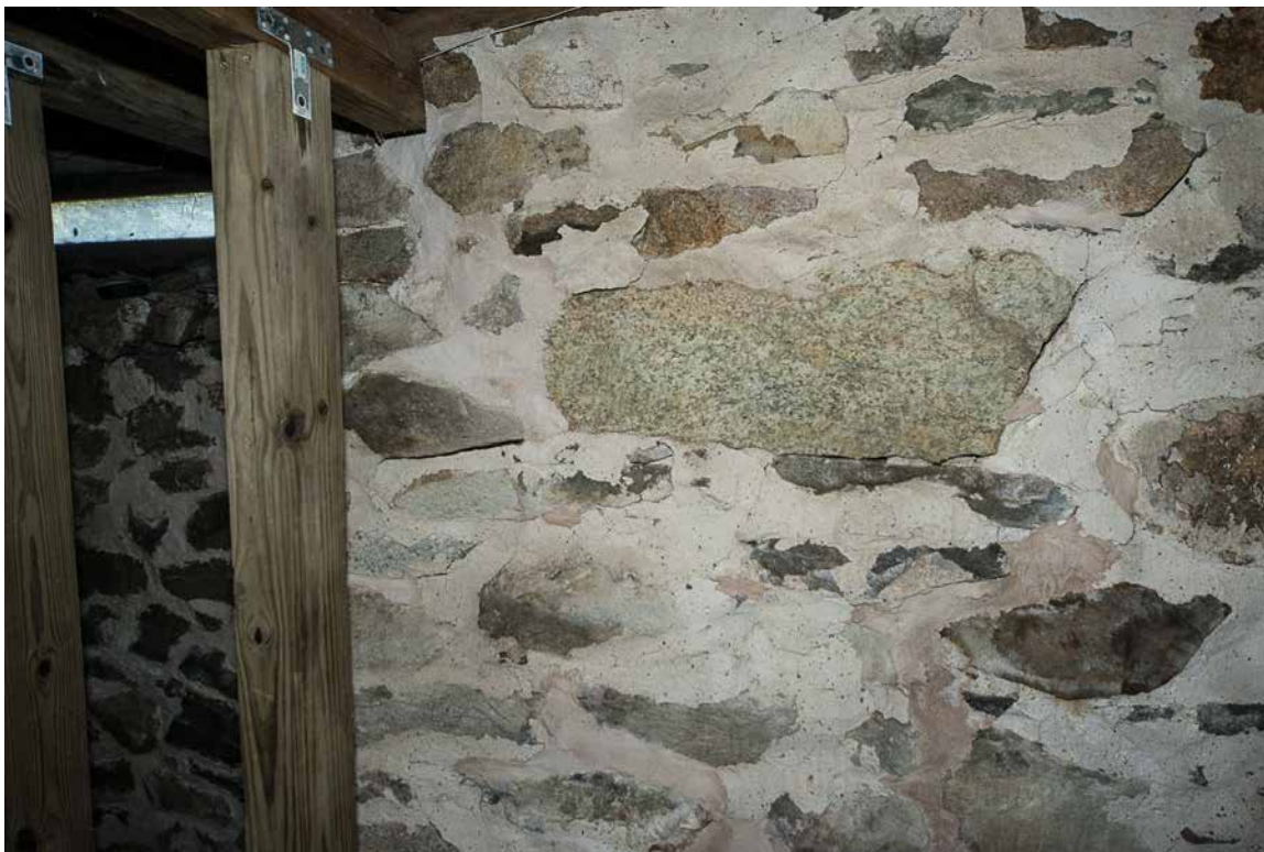
Photo 37: Photo taken in 2016 of the main block cellar below the kitchen showing a small section of its west wall that has some voids in the joints where the mortar butts the stone. The voids due not show up in this photo, but comparison with the 2005 photo shows that both the cracks and the existing mortar predate 2005 and are not a concern.
