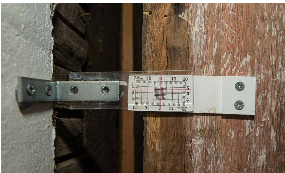
Photo 22: Photo taken in 2016 showing the current position of the red cross hairs on the crack gauge shown in photo 21. The purpose of the gauge was to determine if there is any current movement between the two portions of the building. The slight difference in the position of the cross hairs between the two photos is probably due to the camera angle in photo 21 being slightly off center (above and to the left of the cross hairs) whereas in photo 22 it is straight over the cross hairs. The photos demonstrate that there has been no significant movement over the last ten years and the relationship between the ell and the main block is stable. The original cause of the separation is not known, but it was once covered by a piece of trim that extended from the unpainted portion of the corner post to the plaster lath on the left.
