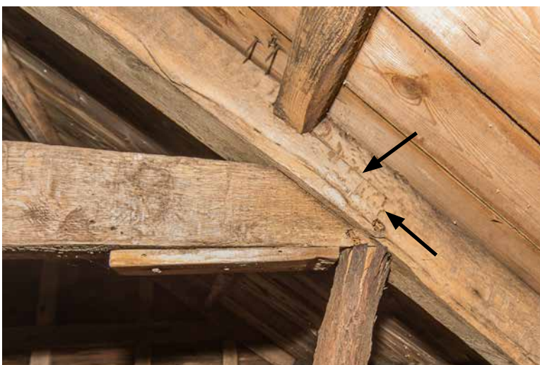
Photo 30A: Junction of rafter tie beam with easterly principal rafter with make-do strut below the joint. The photo is looking toward the north attic gable end. The arrows point to what may be stress cracking. Numerous exit holes in both the rafter and the end of the tie beam indicate past insect activity at this joint. Further evaluation of conditions at this joint is warranted.
