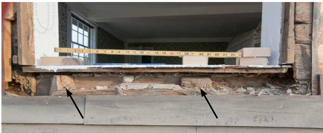
Photo 78: West facade parlor chamber window sill showing evidence that the current two windows in the west wall are not original. They were probably installed when the room was remodeled in the mid 18th century to replace a single window in the center of the wall. The evidence is the two wall studs marked with the arrows that were cut off to install the window. This photo and those below were taken in 2006.
