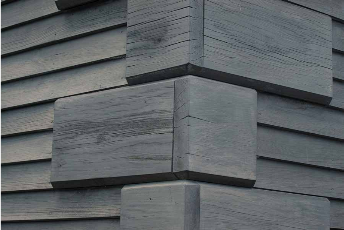
Photo 50: The corner quoins had weather checking in 2005, and the current extent of checking appears to be about the same.
