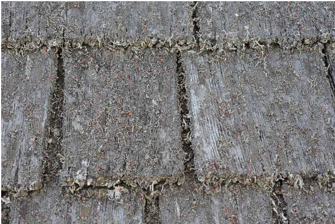
Photo 2: Detail of the front pitch shingles showing the lichen and numerous short splits in the shingles starting at the butts. Dampness is held on the roof by the lichen causing the shingles to rot at their butts.
