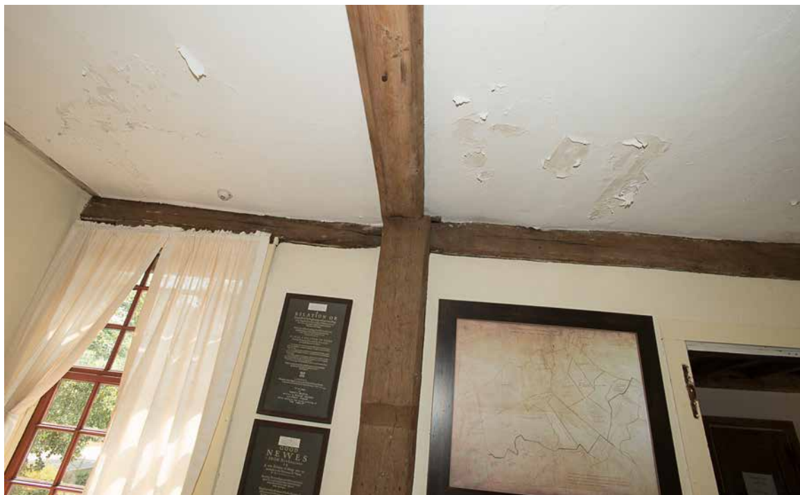
Photo 55: Another 2016 photograph showing substantial paint peeling on the beam casings and plaster ceiling of this room. Other than the parlor chamber, the most substantial peeling was occurring in the rear rooms of the main block.
