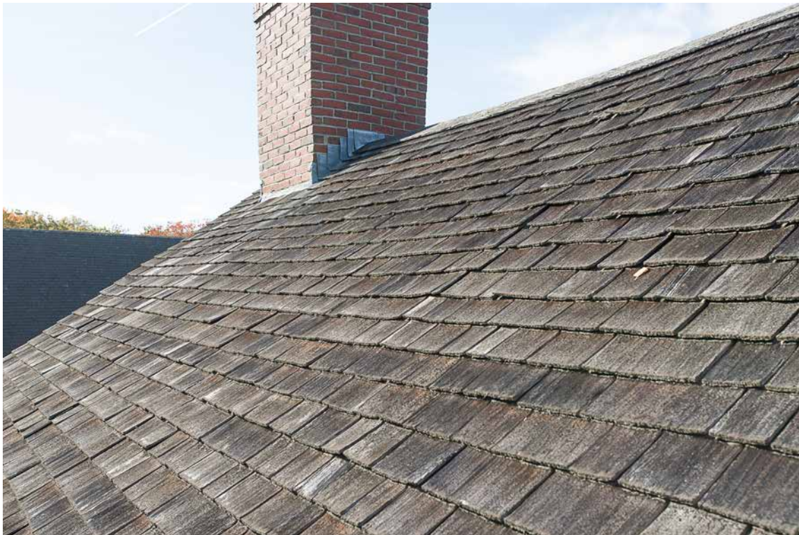
Photo 8: Overview of the south pitch of the rear ell roof and the ell chimney. From this vantage point the shingles appear to be sound, but when examined close up there is considerable wear to the surface of the shingles from ultra-violet (i.e, sun) exposure coupled with erosion from water runoff.
