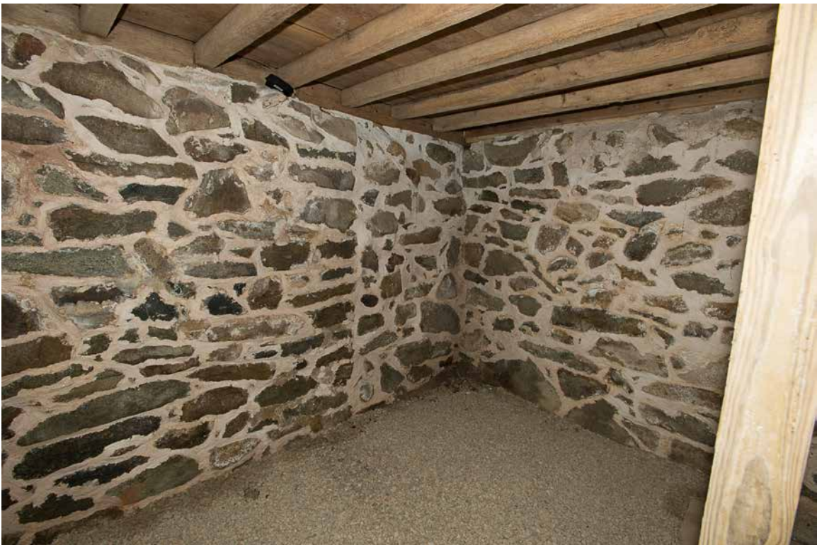
Photo 34: Overview taken in 2016 of the south end (left) and north side (right) of the main block cellar below the kitchen showing the repointing of the foundation done in 2006-7 and the gravel installed over the dirt floor. There are no signs of substantial seepage.
