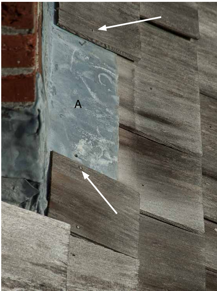
Photo17: Photo taken in 2006 showing the top course of shingles face nailed (arrows) over the lead apron on the downhill side of the chimney and one shingle missing (arrow) with one of its nails sticking out of the flashing and the other leaving a hole in the flashing. Such face nailing can cause leaks. The top course of shingles should be under the flashing with its nails covered by the flashing. If there is a concern about the lead being lifted by the wind, cleats with concealed nailing should be used to hold its lower edge down on top of the shingles. The flashing remains in this condition currently including the missing shingle.
