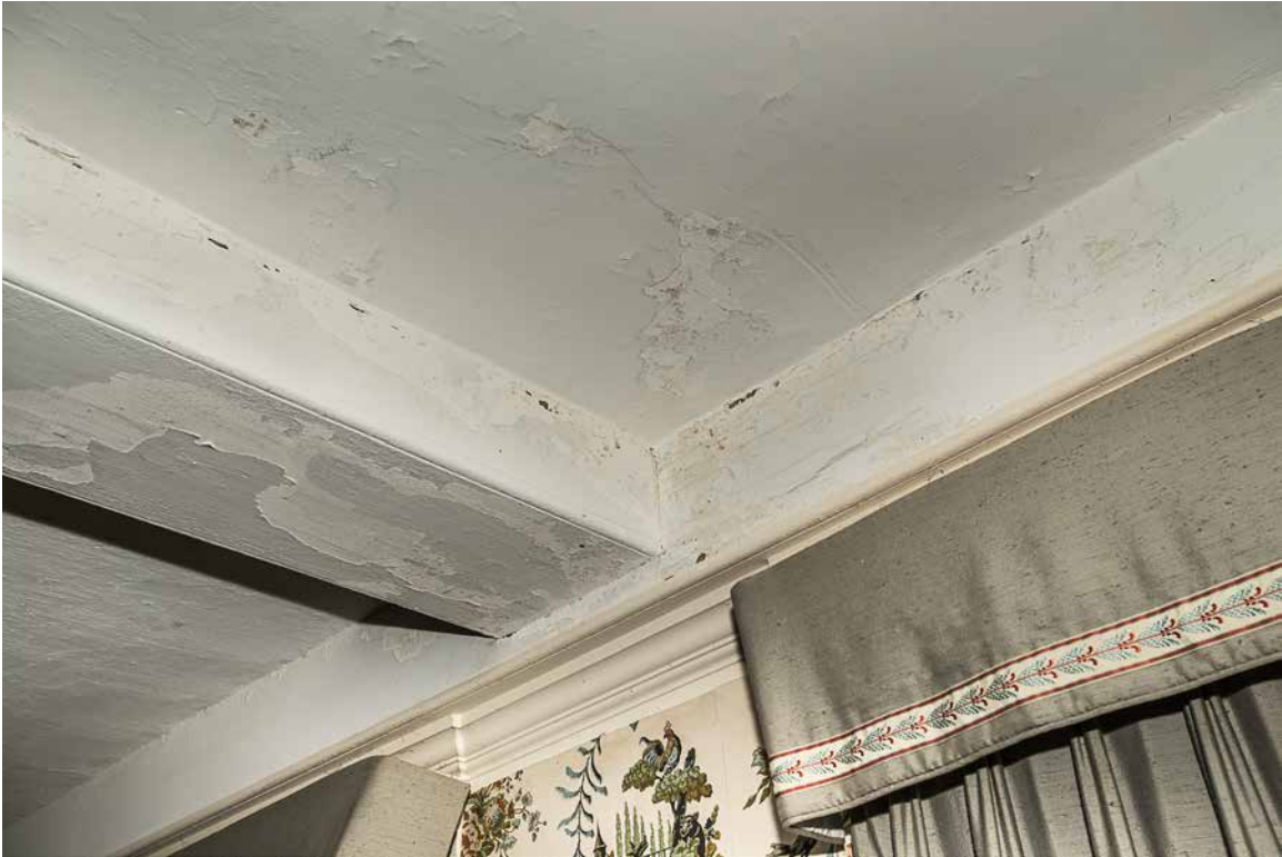
Photo 54: 2016 photograph showing substantial paint peeling on the beam casings and plaster ceiling. While there some paint peeling visible in the 2005 photos, the current extent of peeling is much worse. The primary cause is probably calcimine paint under the current modern paint.
