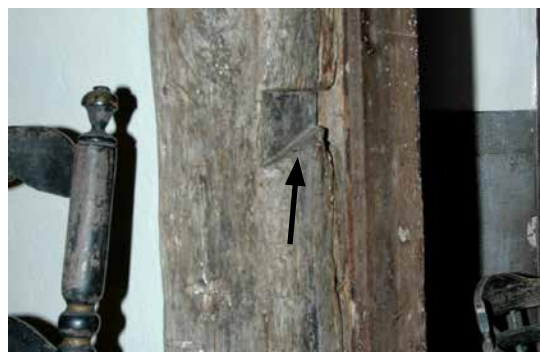
Photo 85: The arrow points to a notch in the left jamb of the door from main block kitchen into the rear ell. The notch probably was cut to receive a bar to secure the back door of the main house before the ell was added, and is further evidence the ell was added later.
