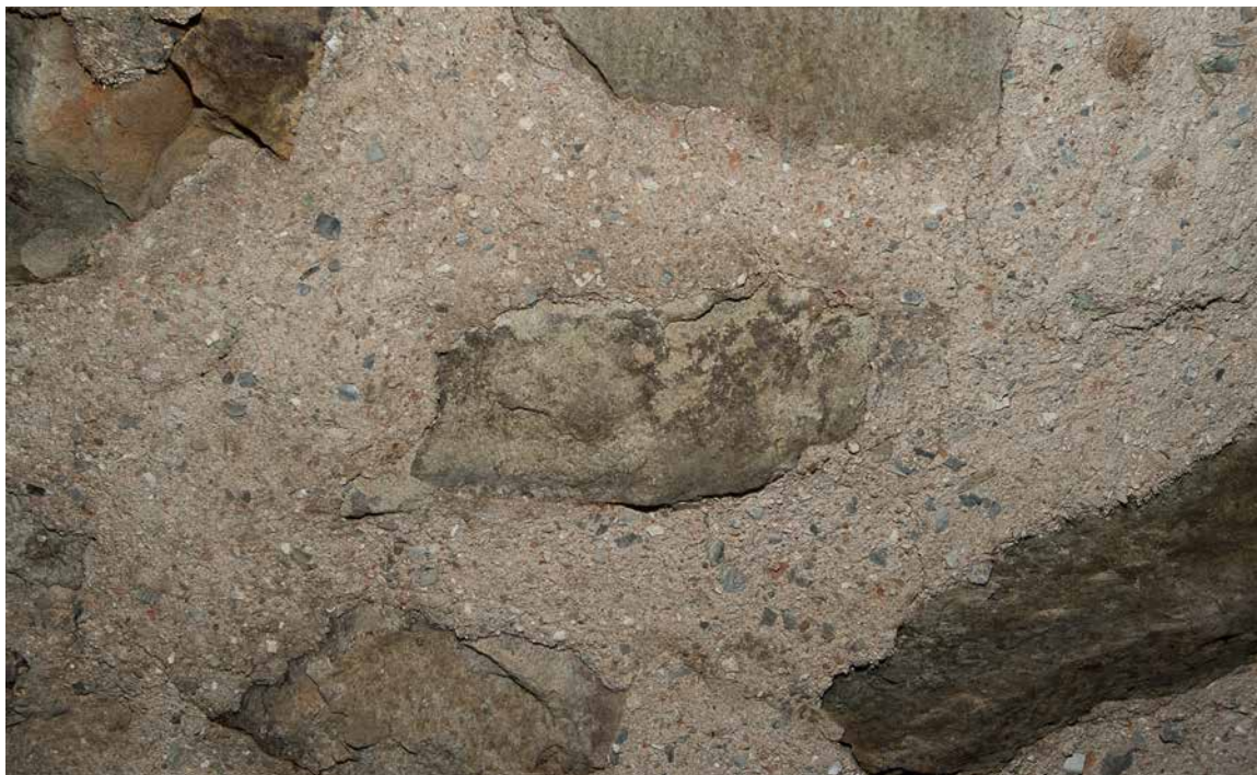
Photo 38: Detail of the mortar joints in the east wall of the main block cellar. The mortar is probably original to the house or very early as it has numerous particles of shells in it that indicate it was made by burning sea shells rather than limestone. It has a distinctive light reddish brown color. As a rare survival of very early mortar it should be retained and preserved. Is is generally in sound condition.
