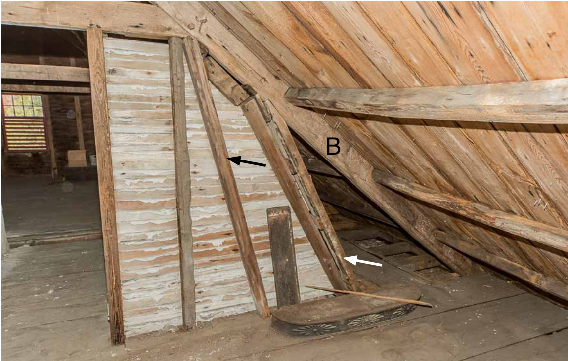
Photo 27: Photo taken in 2016 showing the southerly chimney rafter (B) and the south side of the ca. 1920 attic stair enclosure. The arrows point to an angled post a stud that are seated on the sound portion of the southerly chimney girt. These are probably transferring a significant portion of the roof load from the rafter to the girt. The framing on the south side of the enclosure is similar.
