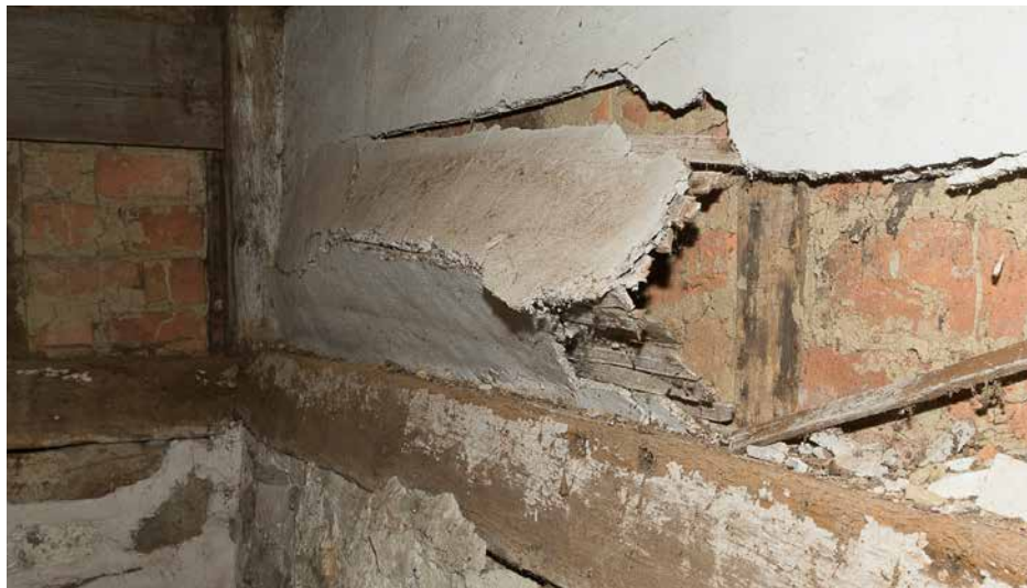
Photo 39: Buckled plaster on the north wall of the dairy. The buckling is more severe than it is in the 2005 photo below. It does not, however, indicate structural issues. It is simply collapsing from its own weight. It could be carefully re-secured to the studs behind it using plaster washers and screws to preserve it.
