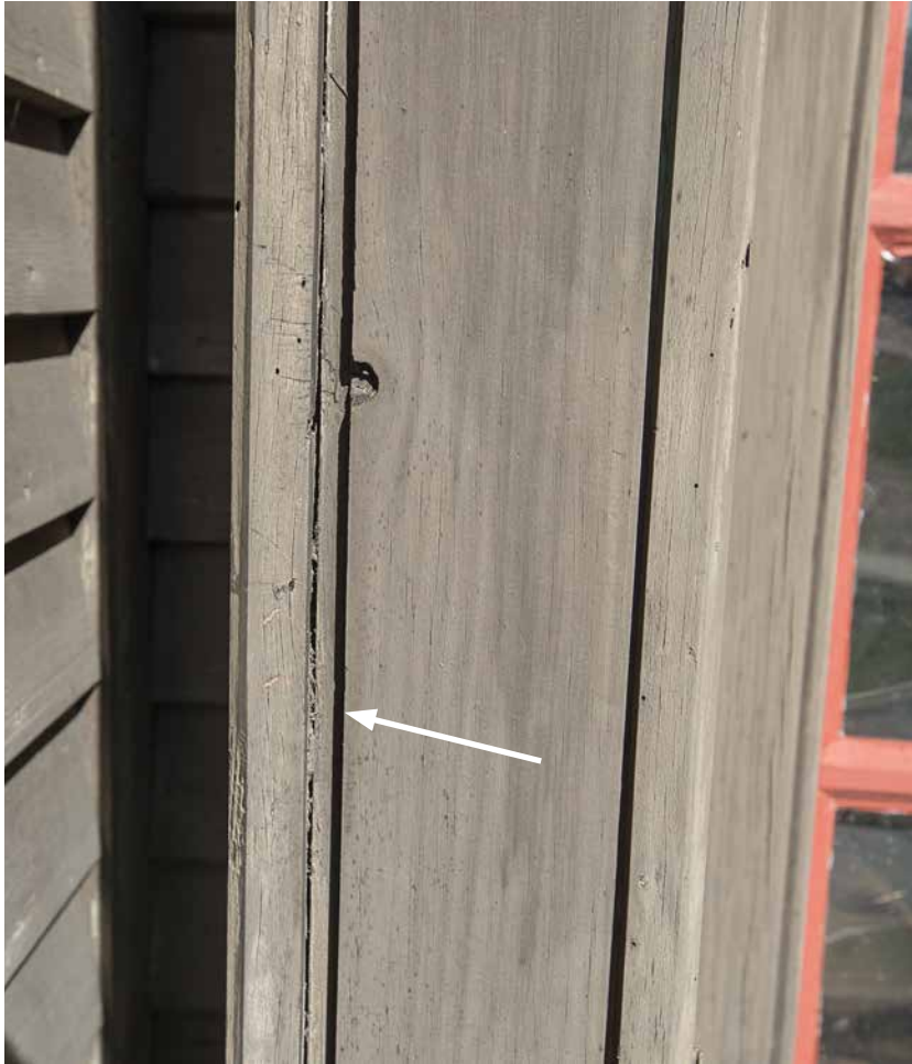
Photo15: The wood downspout casing is coming apart at its seams (arrow). It is not clear why this is happening as there is a copper downspout inside it. This one needs to be taken down , its sides drawn together, and then refastened.
