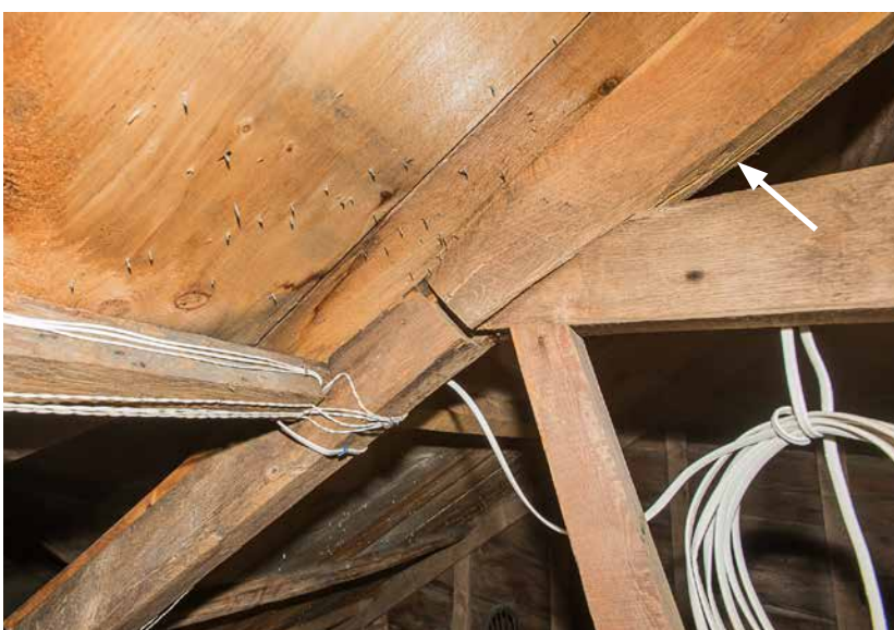
Photo 30B: Junction of rafter tie beam with the westerly principal rafter looking toward the north attic gable end. The portion of the rafter from the bottom of the tie beam upwards appears to be a modern replacement that is spliced to the portion of the original rafter that remains below the tie beam. The arrow points to checks in the underside of the rafter that appear to originate at the splice joint. Further evaluation of conditions at this joint is warranted.
