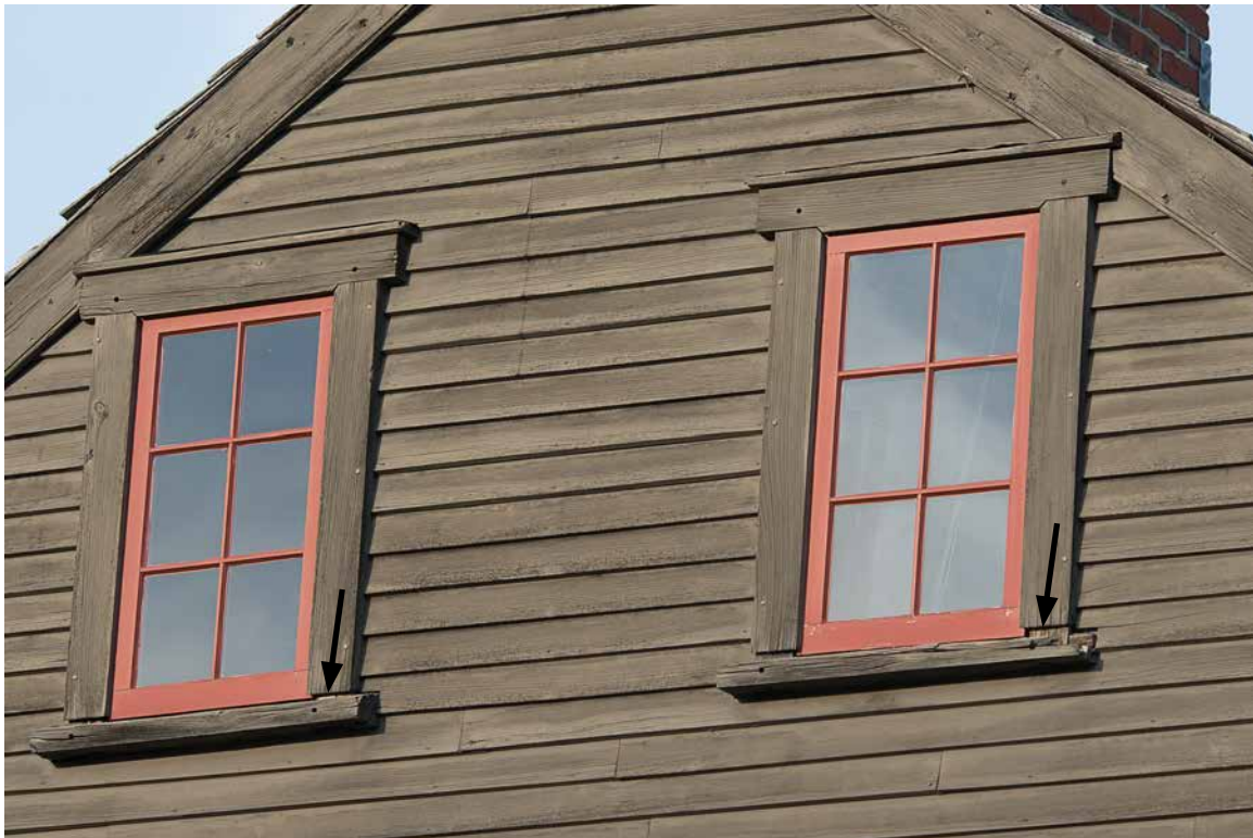
Photo 44: West attic wall of the main block showing two windows where the sills have slipped down exposing the tenons of the jambs (arrows). The frames of these two windows were not repaired in the 2006-7 work, perhaps because access was difficult.
