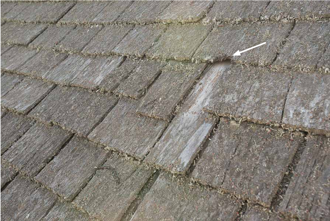
Photo 3: Detail of the front pitch shingles showing one shingle that has slipped off the roof and another slipping down. The arrow points to where the butt end of a shingle is disintegrating from rot. The shingles on this pitch are beyond their useful service life and should be replaced within the next 1-2 yeears.
