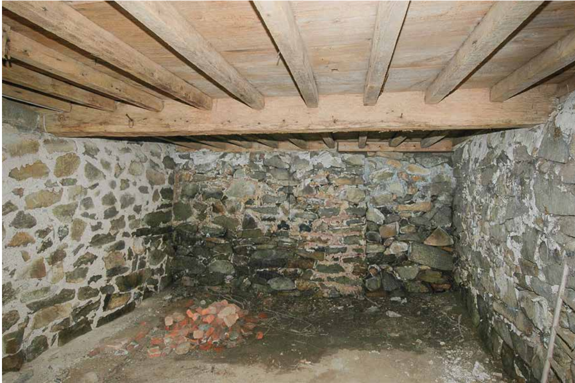
Photo 33: Overview taken in 2005 of the south end of the main block cellar below the kitchen showing excessive moisture seeping into the space indicated by the dark areas on the dirt floor and the foundation wall.
