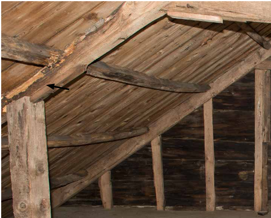
Photo 28: Photo looking toward the south end gable wall showing substantial sag in the common roof purlins as well as past rot in the rafter marked by the arrow. The purlins are undersized by modern standards and their sag has probably been present for many years.
