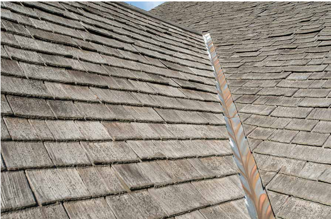
Photo 6: Copper valley between the rear main block pitch (right) and the rear ell south pitch (left). Leaks have been reported in the attic from the area to the right of the valley, but no obvious defects were observed in that area. The shingles on both of these pitches are fastened with stainless steel staples. The ell roof was installed at the same time as the rear main block roof in 1995.
