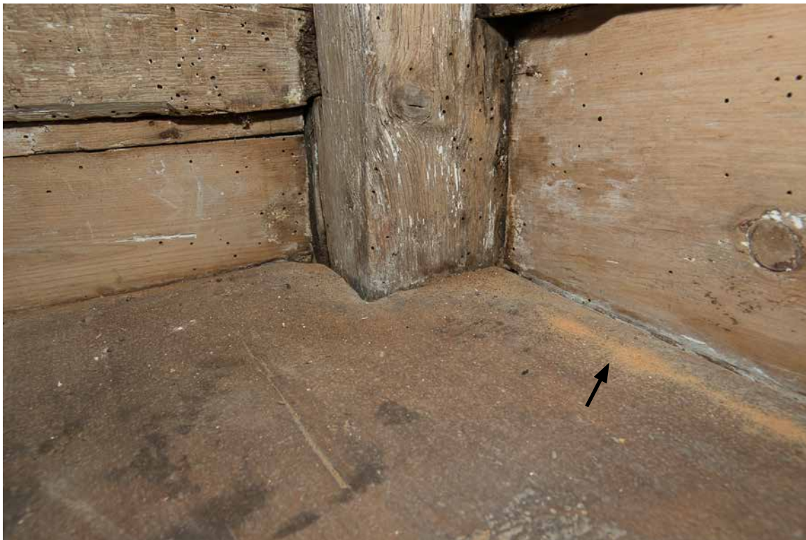
Photo 43: Photo of the northwest corner of the buttery showing recent frass (arrow) from wood boring insects (probably anobia - commonly called powder post beetles). Although has been treated several times since 2005, the insects continue to persist.
