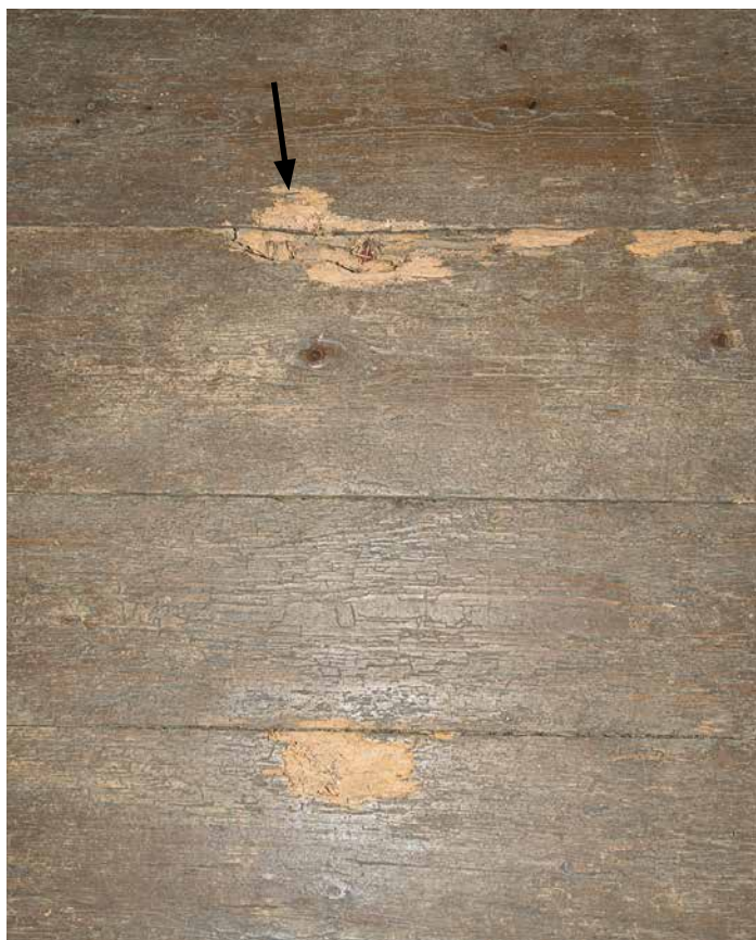
Photo 58: 2016 photo of the same area of damage to the surface of the floor boards in the hall shown in photo 57. The extent of damage has slightly increased since 2005, but is still quite limited.
