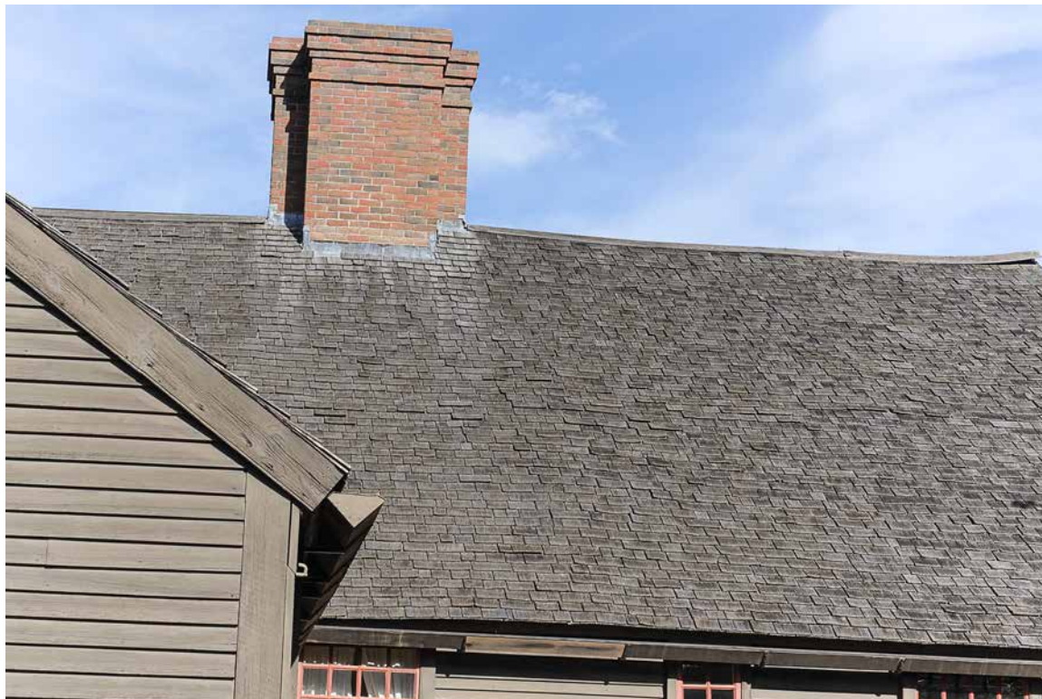
Photo 4: Overview of the rear (west) pitch of the main block roof. These shingles were installed in 1995 using stainless steel staples rather than nails. Some of the staples have come loose, but most are still holding.
