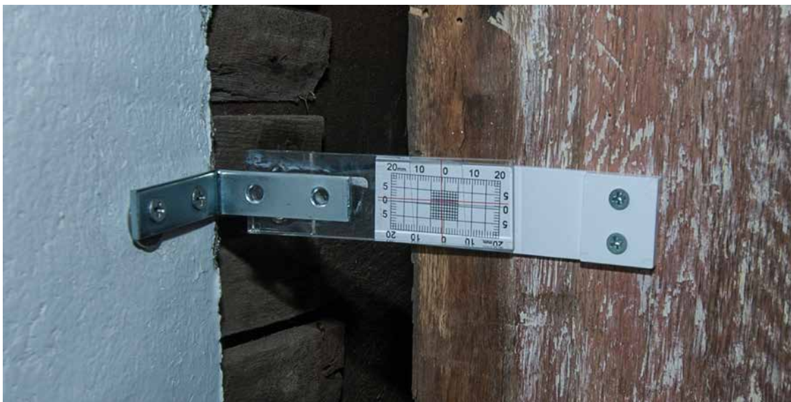
Photo 21: Photo taken in 2005 showing the crack gauge between the main block on the left side and the southeast corner post of the rear ell just after it was installed. The purpose of the gauge was to determine if there is any current movement between the two portions of the building.
