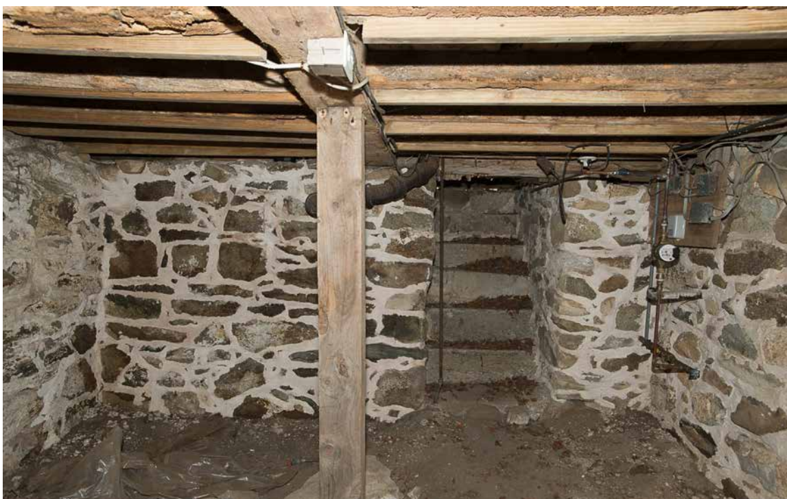
Photo 32: Overview taken in 2016 of the south end of the cellar below the rear ell. The walls were repointed in 2006-7 along with rebuilding the bulkhead cover and adding gutters below the roof. The soil was dry and there were no signs of seepage through the foundation wall. Examination by Peter Krusell after periods of heavy rain did not show any signs of seepage. That the data logs recorded this year still showed high relative humidity is probably a function of vapor transmission from the soil and the foundation walls.
