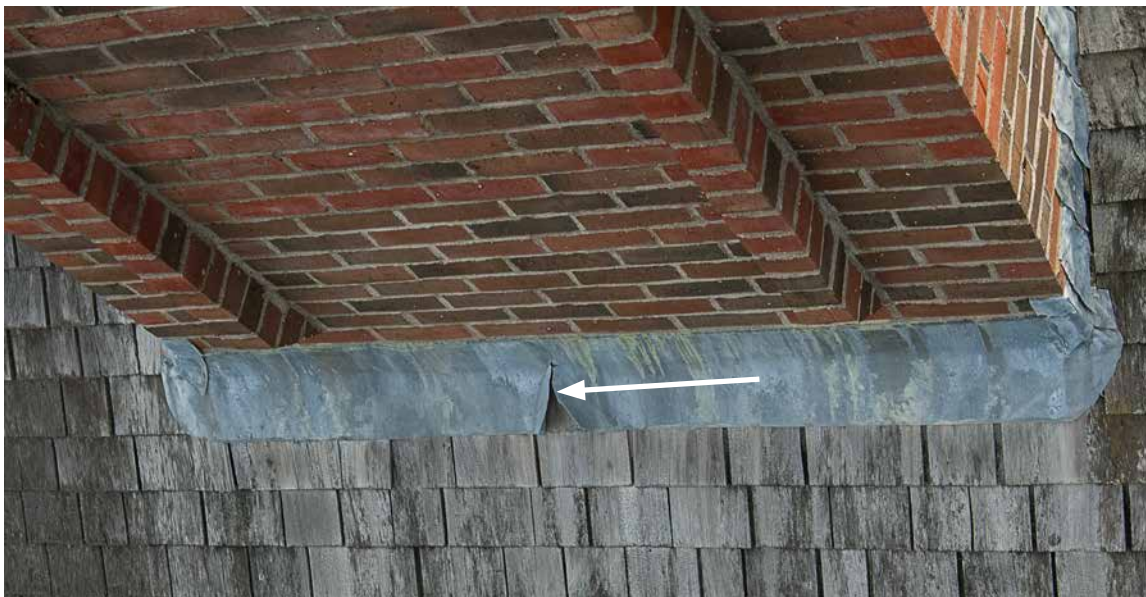
Photo18: Photo taken in 2006 showing a large tear (arrow) in the lead apron flashing on the front side of the chimney. The tear was probably caused by fatigue failure from thermal stress in the long strip of 2 1/2lb. lead. Long exposed pieces of lead should be done using 4 lb. lead to avoid fatigue failure. The flashing remains in this condition today.
