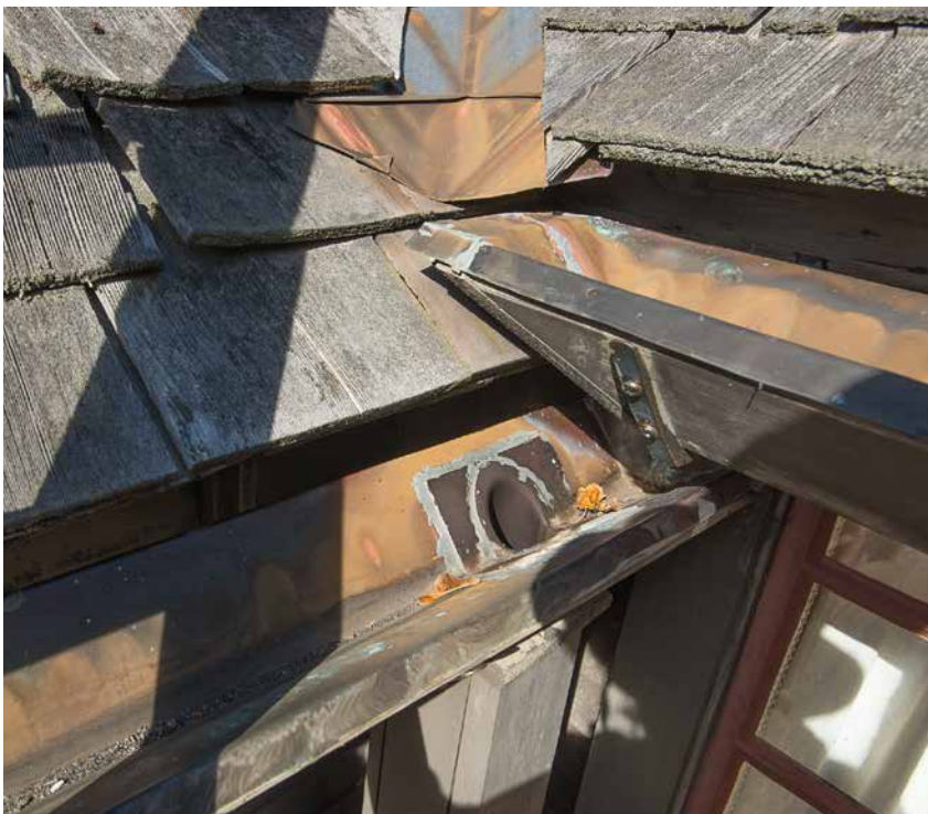
Photo14: gutters showing the top of the downspout. When cleaning the gutters the downspouts should also be checked and cleared of any debris.
