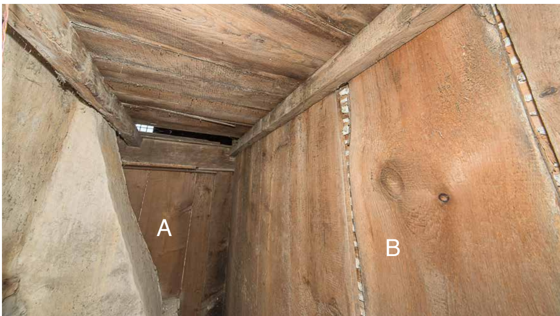
Photo 67: The interior of the space around the chimney looking from the hall chamber end towards the parlor chamber fireplace wall (A). The back wall of the main staircase is on the right (B). It is somewhat curious that these walls are framed with boards rather than studs. That the gaps between the boards are fairly wide indicates that they did not form the finish to the staircase or the parlor chamber. The lath and plaster on them date to the 18th century as the lath are clearly riven and of uneven width and may be the original finish.
