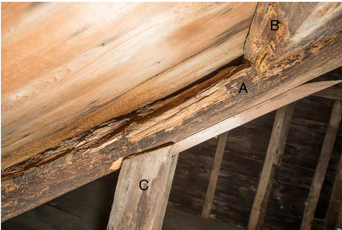
Photo 29: Detail of the rafter (A) marked with the arrow in photo 28 and the purlin that passes over it (B). The strut marked “C” was added some time ago to help support the damaged rafter. The upper third of the rafter is severely rotted, as is the purlin where it passes over the rafter. As the roof sheathing does not show rot above the rafter, the damage must have occurred prior to the installation of the current roof sheathing.
