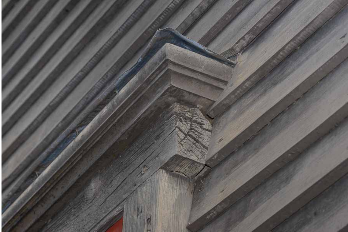
Photo 51: The weather checking in th window head does not appear to be worse than it was in 2005. The metal flashing on top of the cap needs to be tacked down tight to the cap.
