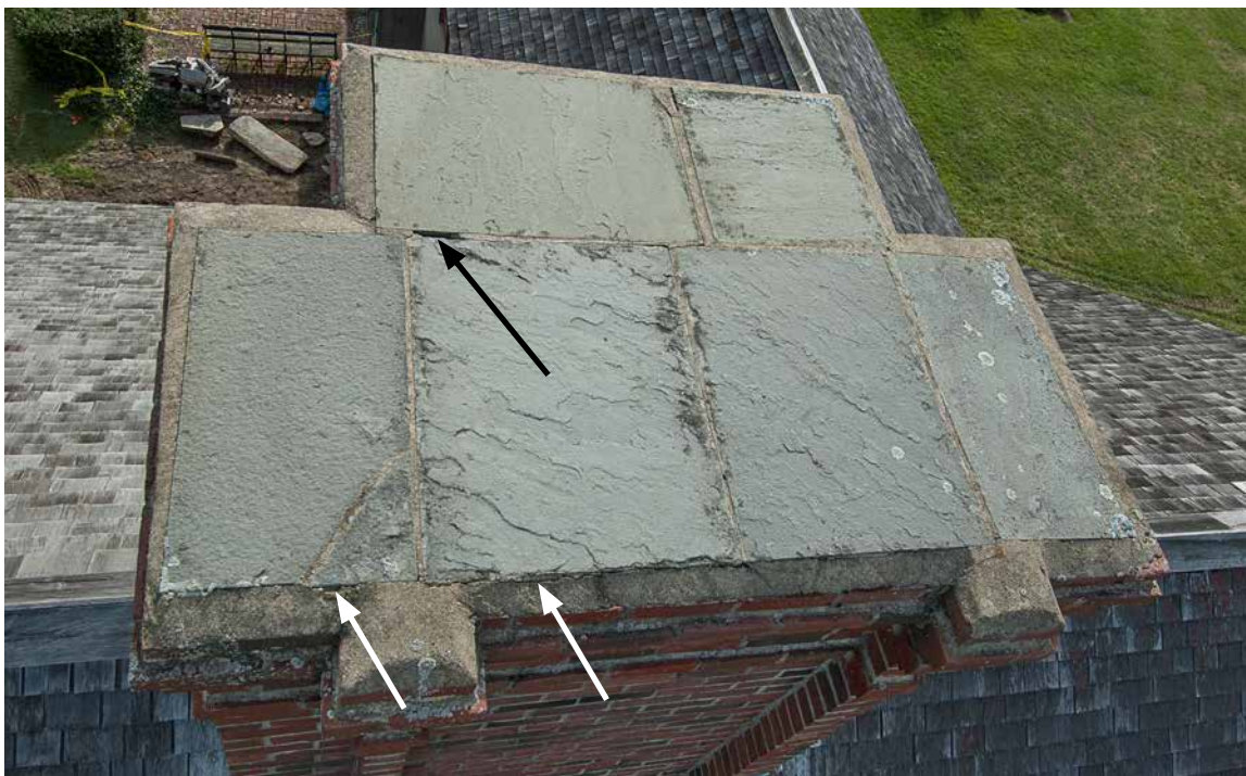
Photo19: Photo taken in 2006 showing the bluestone cap on the main block chimney. The white arrows point to hairline separations between the mortar and the bluestone, the black arrow points to a void in the mortar joint. These defects are probably now worse and can allow water infiltration into the chimney flues. The cap should be inspected when the roof is replaced and defective mortar joints redone. Each piece of bluestone is likely over an individual flue. Replacing a couple of bricks with ventilator bricks would help prevent excessive moisture penetration into the flues due to high internal humidity.
