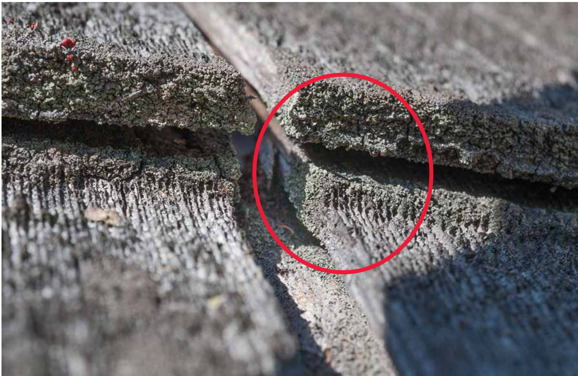
Photo 10: Close up detail of the south pitch of the rear ell roof shingles showing the extensive surface erosion starting abruptly below the butt line of the course above (circle).
