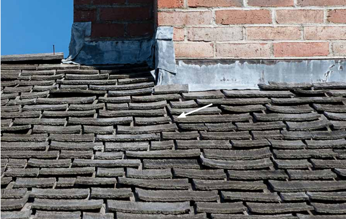
Photo 5: Detail of the rear pitch. Arrow points to one of several places on this pitch where the vertical joints between shingles are in alignment for three successive courses in violation of normal installation standards. Such alignment can generate roof leaks.
