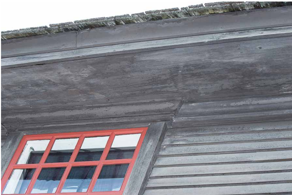
Photo 49: The underside of the front roof soffit is very blotchy indicating it needs to be repainted.
