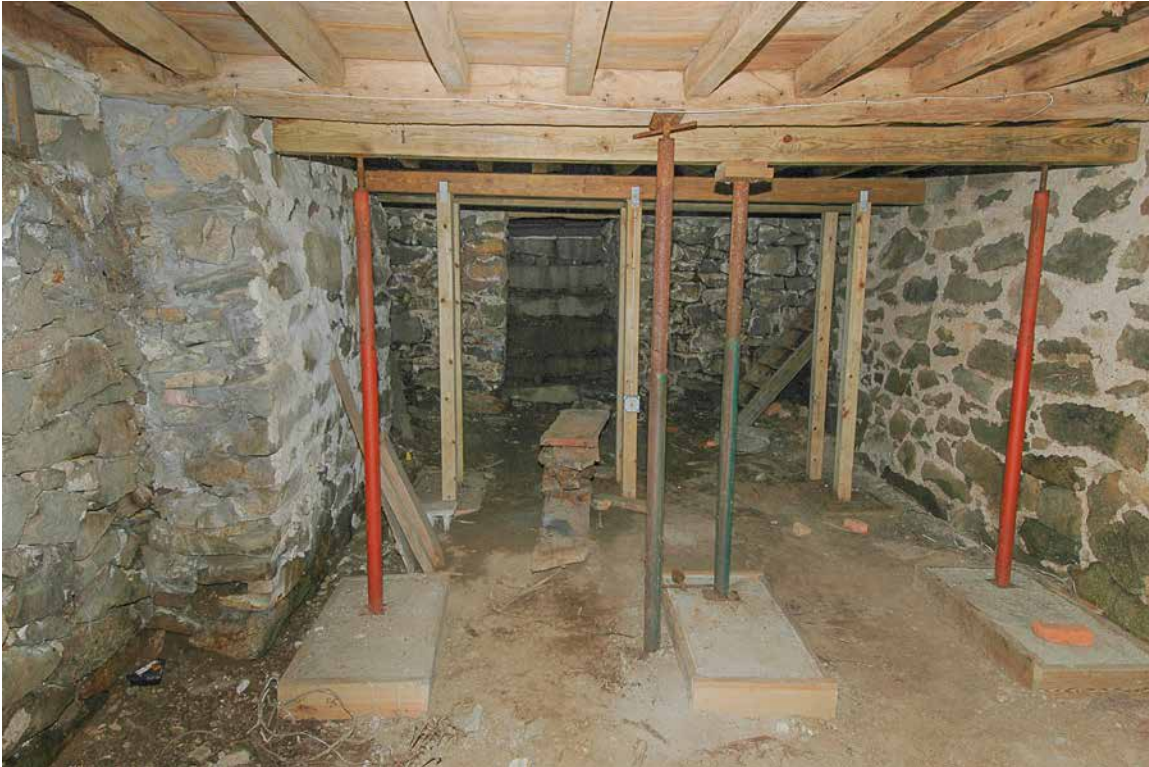
Photo 35: Overview taken in 2005 of the main block cellar below the kitchen looking towards its north end. Dark areas on the dirt floor indicate excessive moisture seeping into the space. Some of the support for the ceiling framing is provided by metal screw jacks which are not considered stable for long term support.
