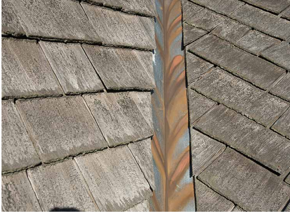
Photo 7: Detail of the copper valley in photo 6. The orange areas indicate wear to the copper from water running off the shingles, but there are no holes from the wear. Pushing on the copper at the wear spots indicated the wear is currently very minor.
