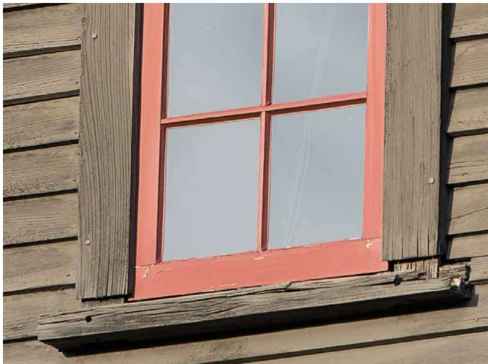
Photo 45: Detail of the southerly window showing that the sill has partially rotted away around the tenon of the right side jamb. This sill needs to be replaced.
