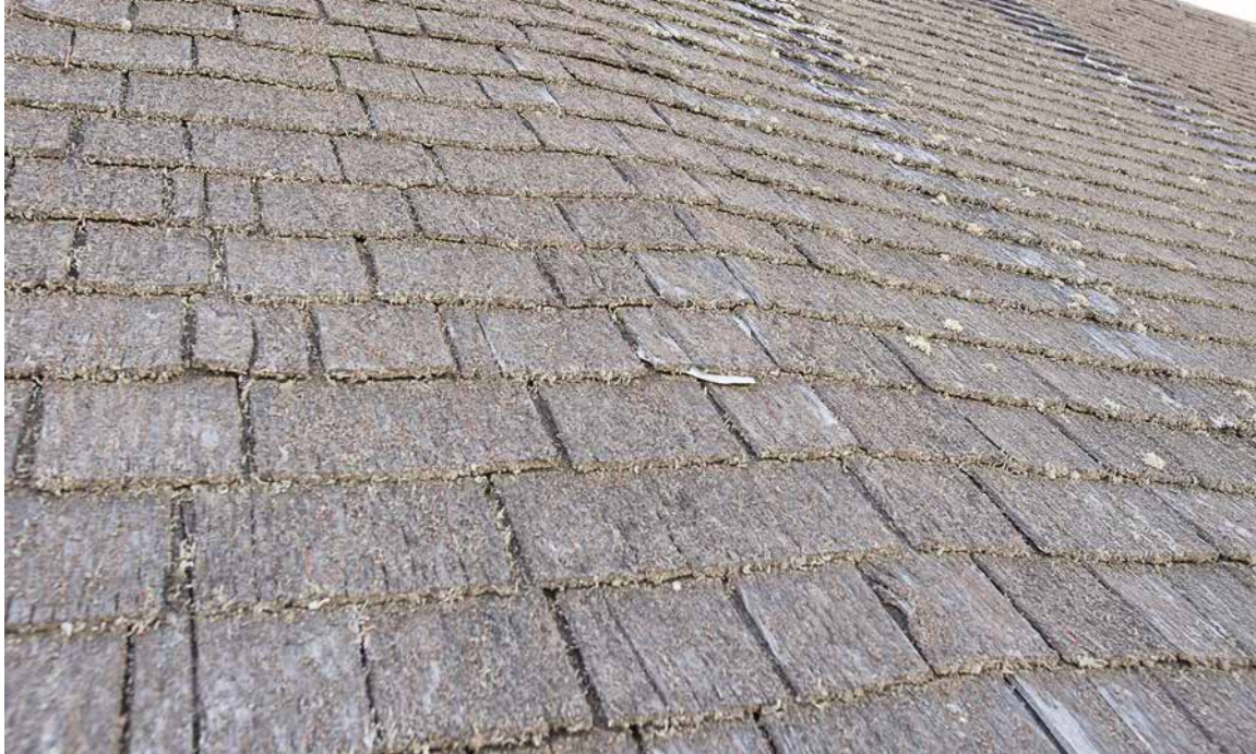
Photo 1: Overview of the front (east) pitch of the main block roof showing extensive lichen growth on the shingles. There is a hump where the shingles are over a principal rafter with a visible sag on each side of the hump that follows the existing sag in the purlins and roof sheathing. In installing new shingles the abruptness of the hump could be smoothed out with graduated shims on the sheathing at each side of the rafter. The shingles on this pitch were installed in 1988 using galvanized nails and are at the end of their service life.
