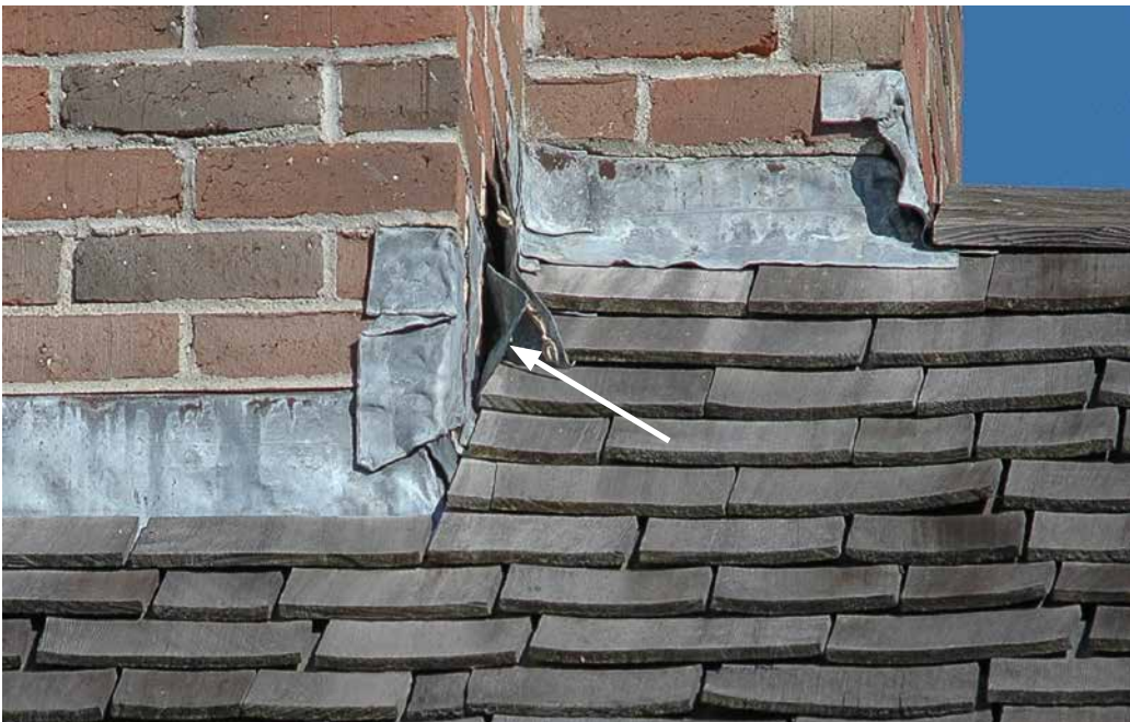
Photo16: Photo taken in 2006 showing the chimney flashing not properly seated against the chimney. Their condition is currently unchanged.
