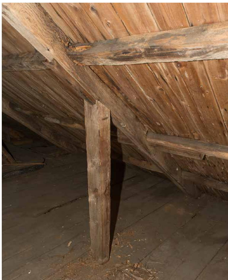
Photo 30: Overview of the damaged rafter and purlin in photo 29 showing the strut (C) that been added to carry loads from the weakened rafter down to the girt under the floor boards. While it probably has prevented failure of the rafter, it does not prevent future failure of the purlin where it passes over the rafter. The conditions at this location should be evaluated by a carpenter with substantial experience repairing 18th century timber framing and repaired as needed.
