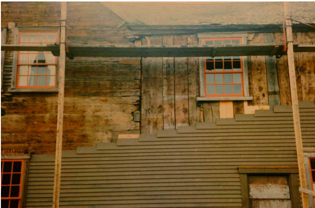
Photo 84: Junction of the north sides of the main block and the rear ell during the installation of new clapboards in the 1990s. The sheathing on the main house runs horizontally indicating it is of stud frame construction. The sheathing on the ell is vertical indicating it is of plank frame construction. Using a different framing style makes the ell unlikely to have been built as an original part of the house.
