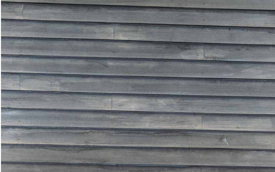
Photo 48: Clapboard siding where the paint (actually a semi-opaque stain) has weathered to become thin and blotchy, and no longer provides adequate protection to the wood surface against deterioration from ultra-violet light and moisture.
