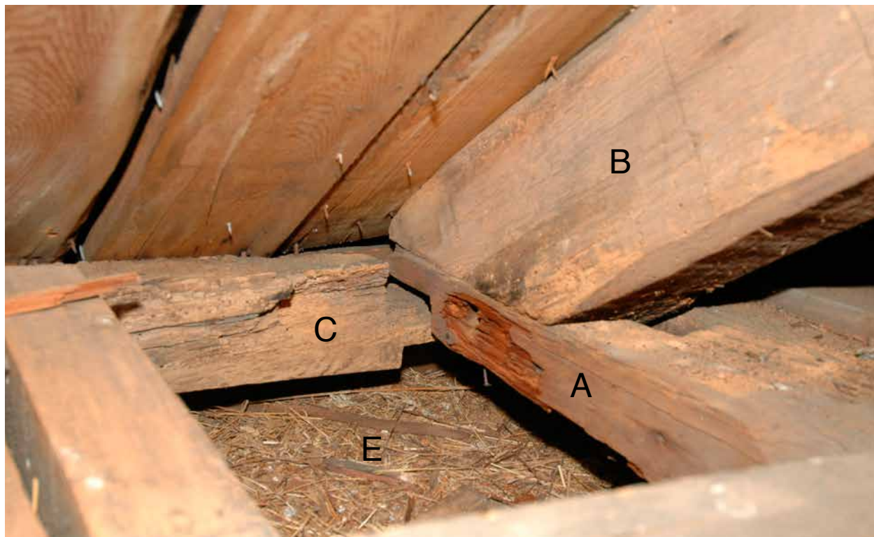
Photo 23: Photo taken in 2005 of the end of the southerly chimney girt (A) and rafter (B) above the front entry. “C” is lowest common purlin that carries the bottom of the roof sheathing over the roof cornice and soffit. The debris at “E” is on top of the cornice soffit. The bottom half of the girt has rotted away.
