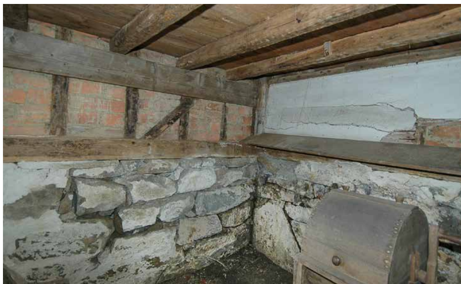
Photo 40: Photo of the north (right) and west walls of the dairy in 2005 showing the buckled plaster on the north wall. The mortar joints in the foundation wall are severely eroded.
