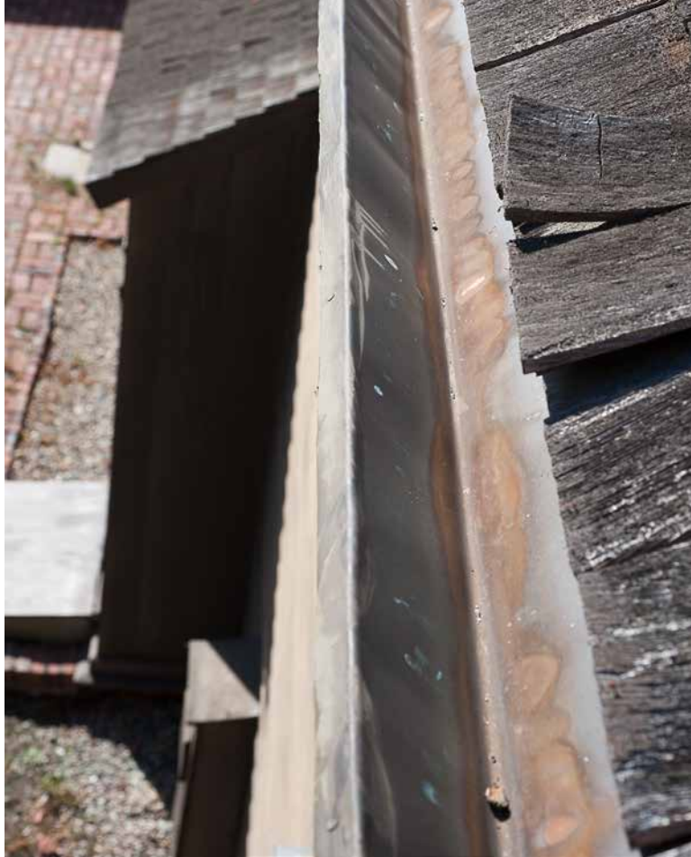
Photo13: The gutters installed in 2007 remain in sound condition and were clear of organic debris at the time of our site visit in October. It is important that they be inspected and cleared of any organic debris on a regular basis.
